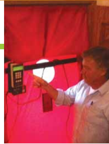
Larry Johnson of LJ Weatherization performs blower door testing as part of an HEA with Building Diagnostics.
