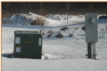
Pad-mounted transformer with lot line meter pedestal
