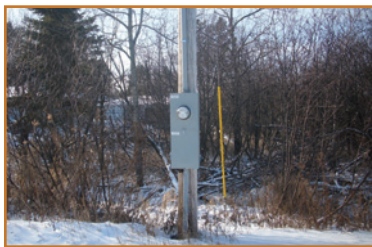
Meter enclosure on power pole
