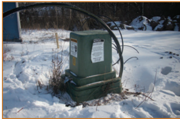
Secondary pedestal with conductors
