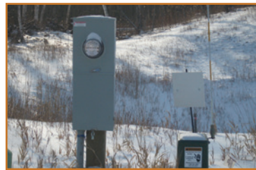
Secondary pedestal with meter pedestal
