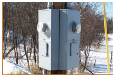
Meter enclosures on power pole
